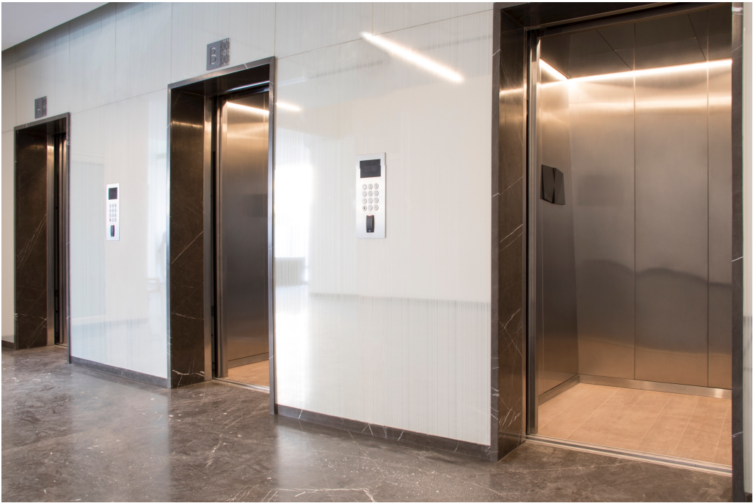
Three different views of all three elevators
